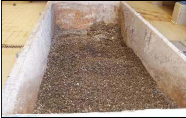
Figure 34: Sewage Treatment Plant Sands
