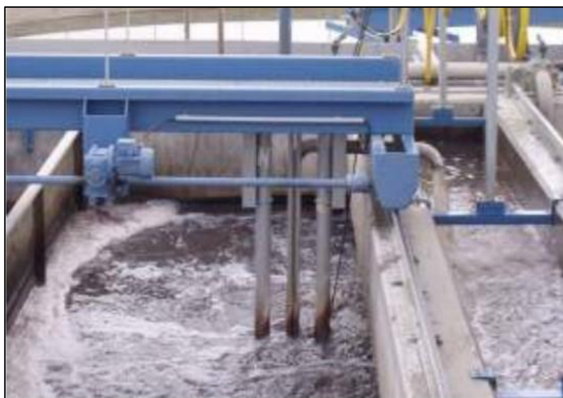
Figure 35: Grit and Grease Separator
